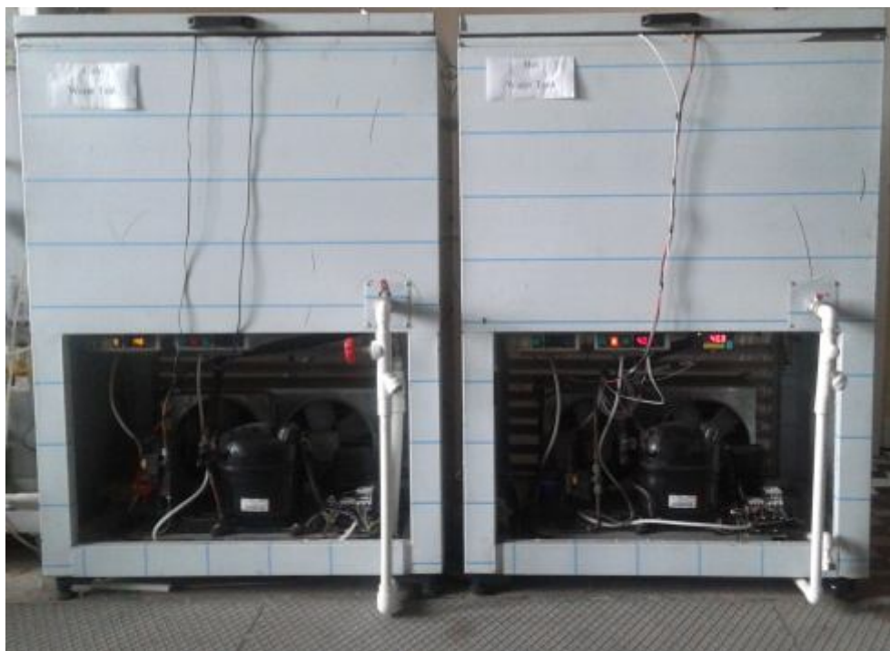
Figure 3.13 Hot and cold water production tanks
