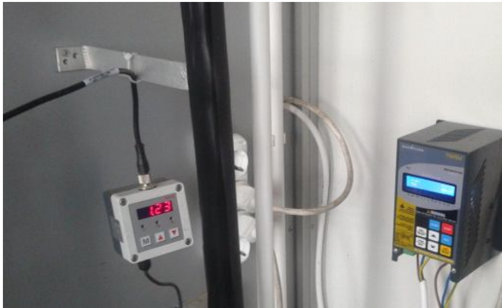
Figure 3.12 Flow meter and frequency controller of pump
