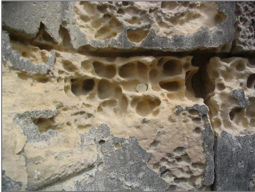
Figure 2.11 Honeycomb weathering on St Etienne church, Fecamp, Seine-Maritime, France (limestone). This church is located 300m of the sea (Angeli, 2007).
