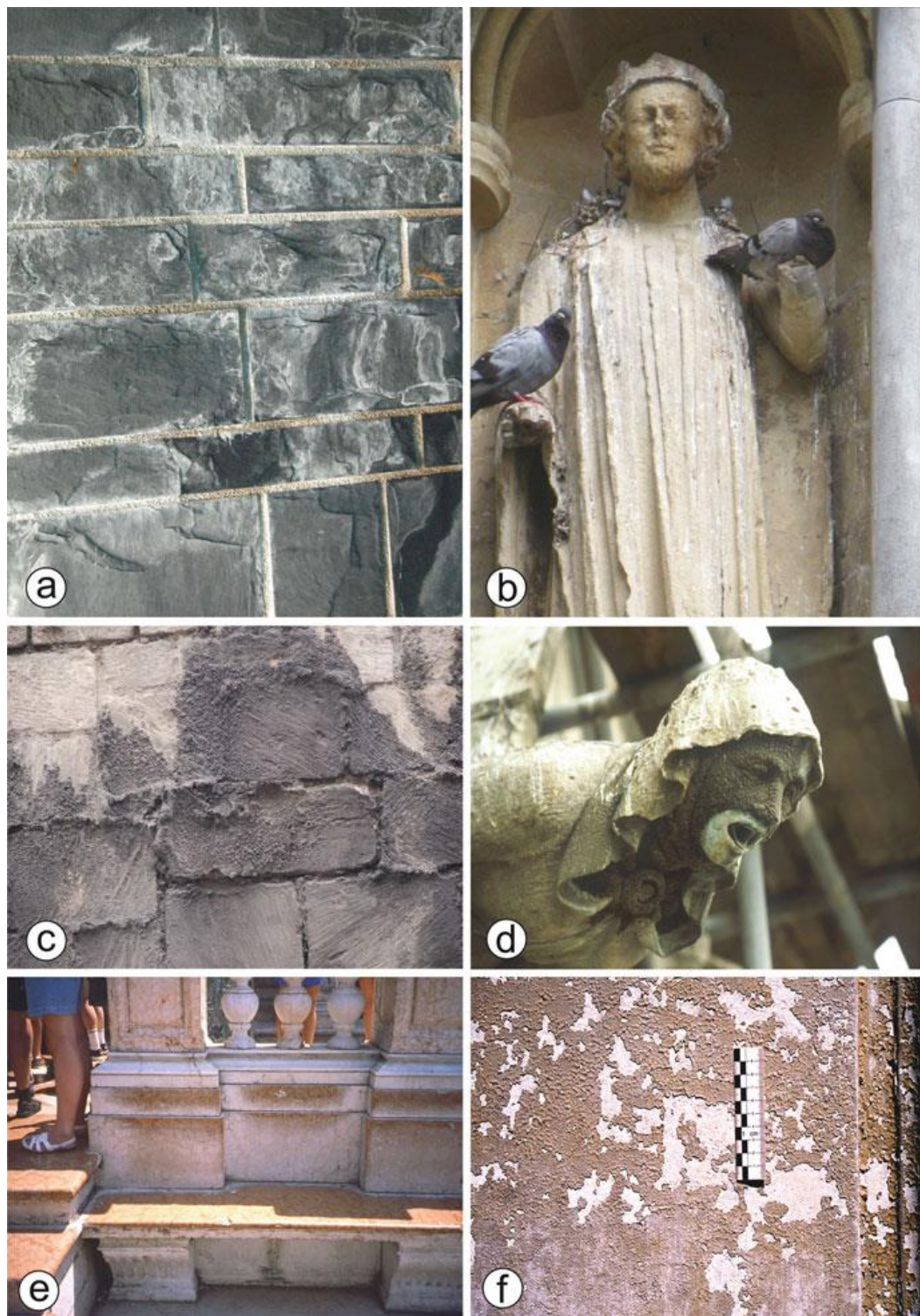
Figure 4.7 Discoloration and deposit 1: (a) encrustation on slate (Germany), (b) deposit of pigeon droppings (U.K.), (c) gypsum crust (Germany), (d) gypsum crust (Germany) (e) bleaching and glossy aspect (Italy), and (f) film: old oil paint on sandstone (Germany) (Siegesmund & Snethlage, 2011)
